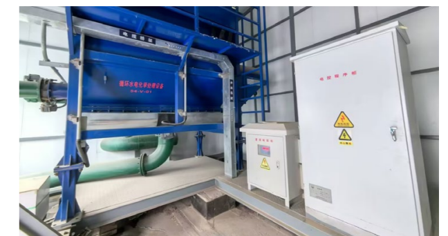
Water-Saving Process Equipment
